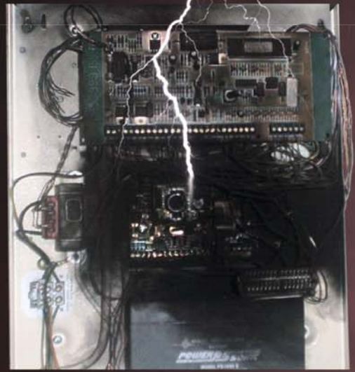
Hazard alert system destroyed in a thunderstorm
